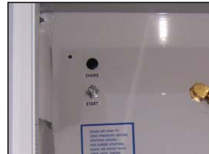
Remote engine controls in right front compartment.
